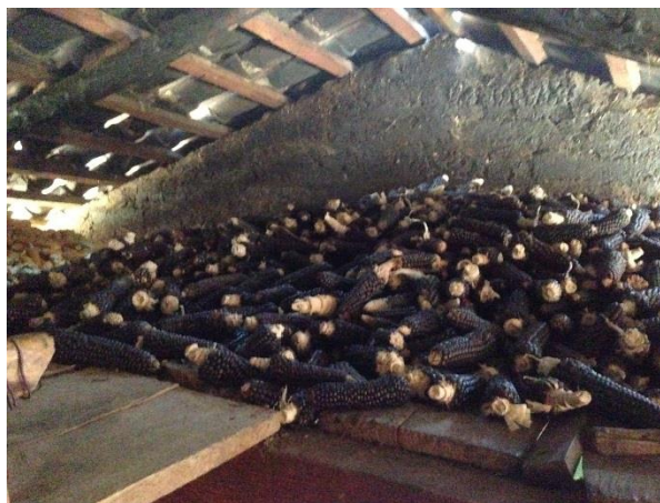
Attic (accumulated heat & sun) or on top of the roof
