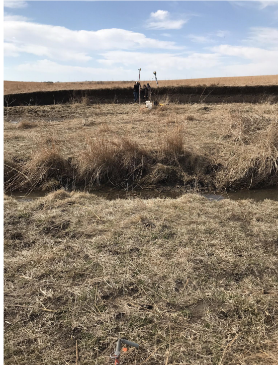
Figure 3: Below is the cross section view at Site 1, looking towards right bank.
