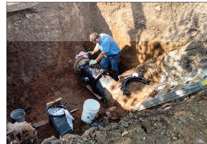
A worker repairs the water main valve to restore the water supply to the KSU Gardens. More information in the Director's column on page 2.
