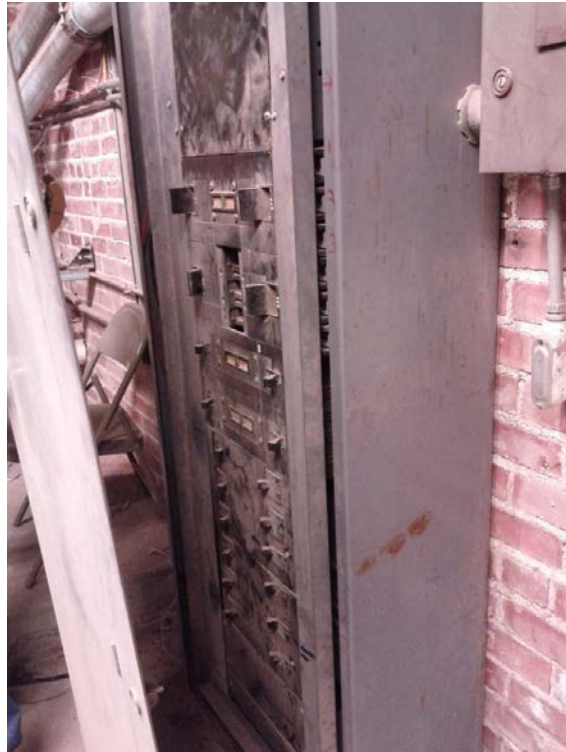
Military Science – Service Entrance Panel outdated and not code compliant.
