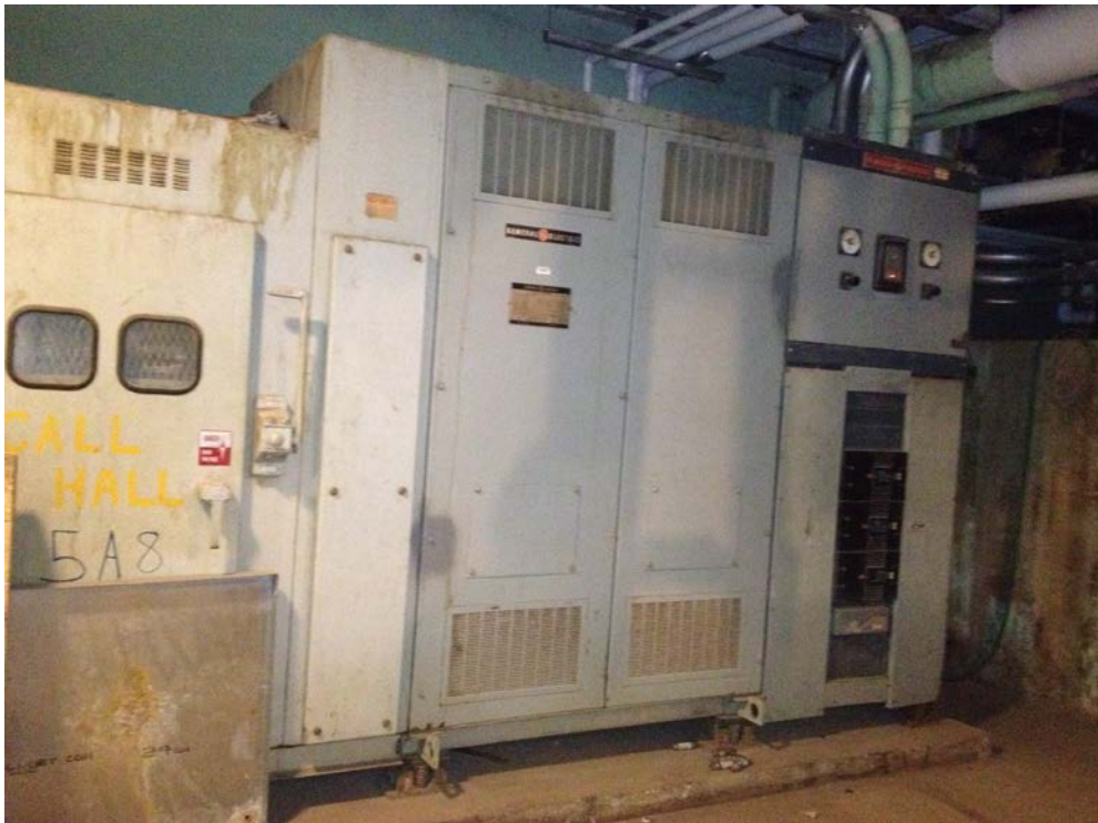
Call Hall – Outdated Unit Substation.
