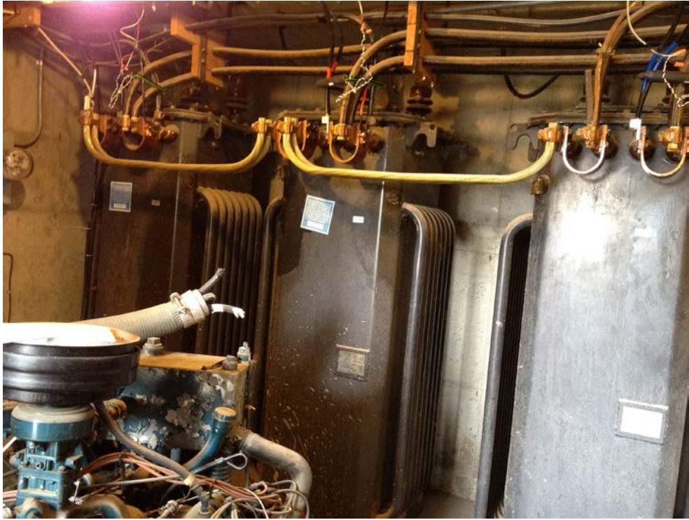
Ahern Field House – Outdated and Non-Code Compliant Transformer.
