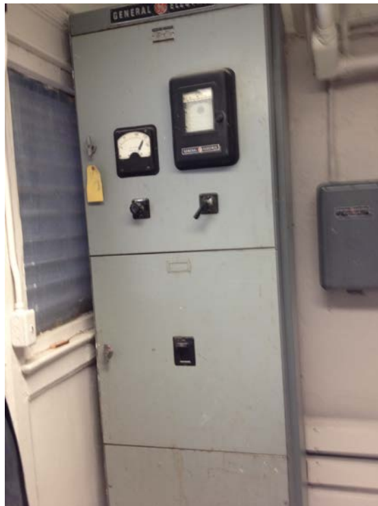
Leisure Hall – Service Entrance in Common Hallway. Clearance space not code compliant.
