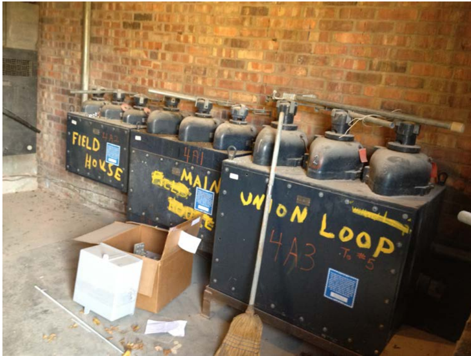
Ahern Field House – Outdated 4160-volt switches.
