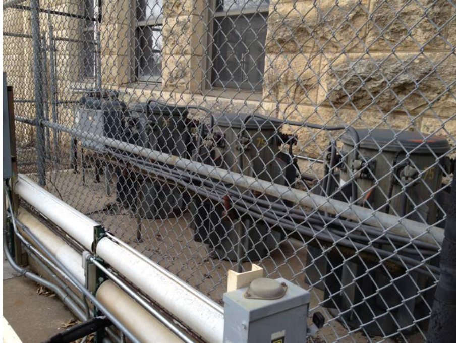
Leisure Hall – Outdated Equipment and Non-Code Compliant Transformer.
