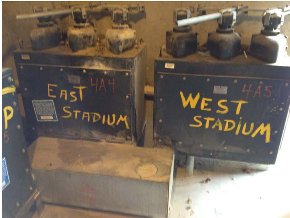
Ahern Field House – Outdated 4160-volt switches.
