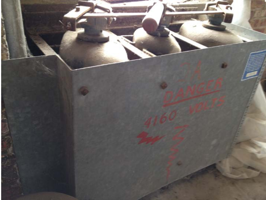
Power House - Outdated 4160-volt switches.
