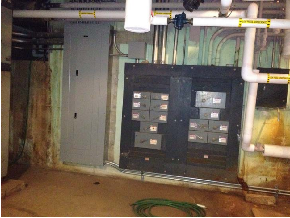
Call Hall – Outdated electrical equipment.
