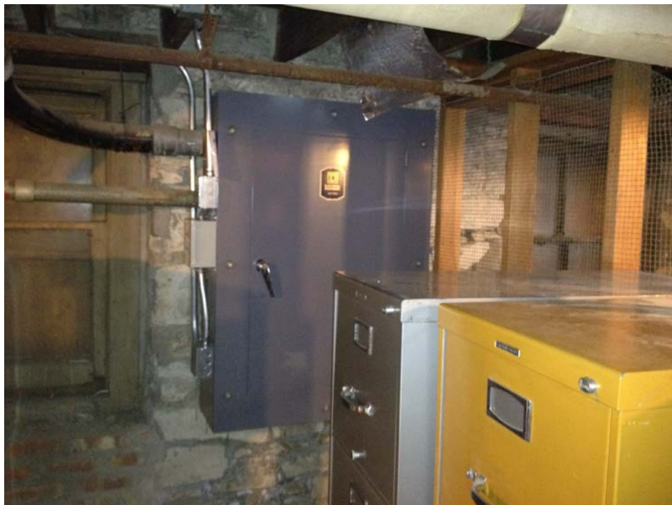
Eisenhower Hall – Clearance space not code compliant.
