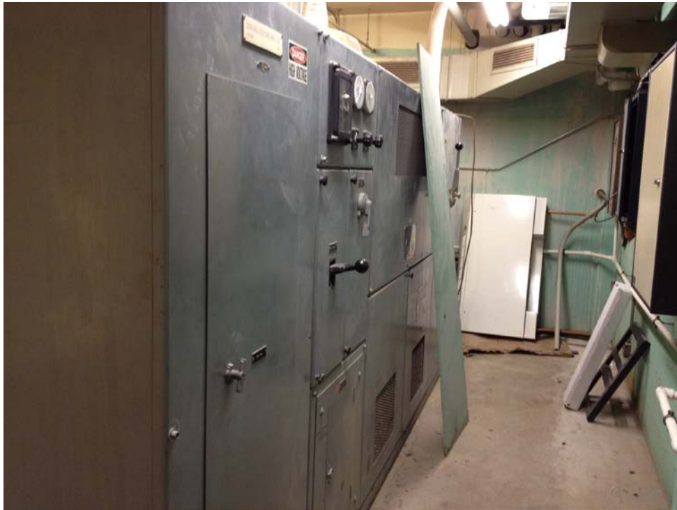
English/Counseling Services – Outdated electrical equipment.
