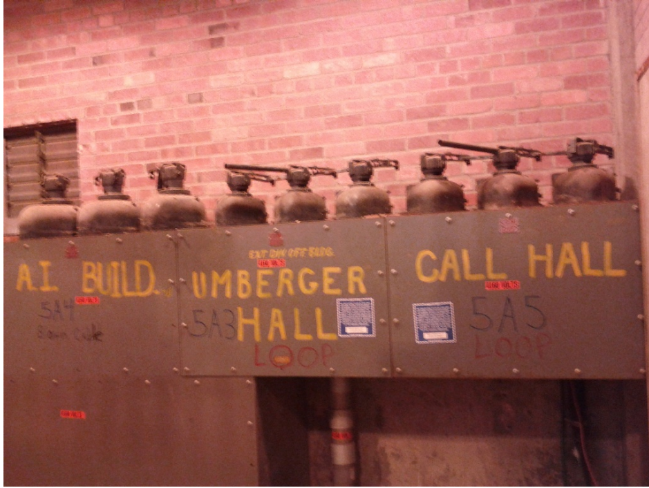
Umberger Hall – Outdated 4160-volt switches.
