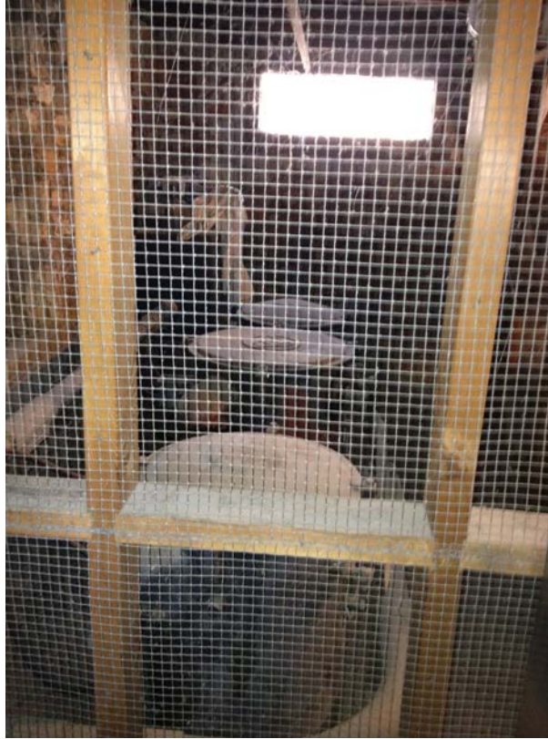
Eisenhower Hall – Outdated and Non-Code Compliant Transformer.
