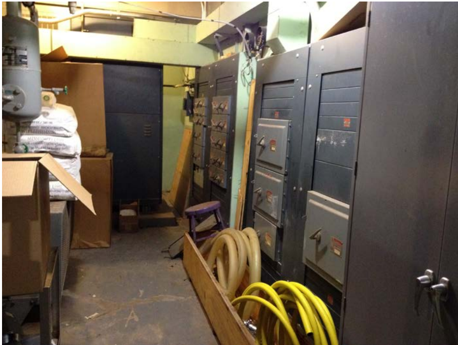
Call Hall – Outdated electrical equipment. Clearance space not code compliant.
