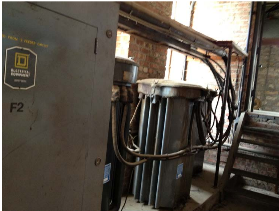
Power House - Outdated equipment and Non-Code Compliant Transformer.
