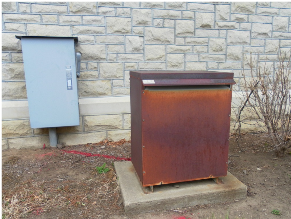
Campus Creek – Undersized Transformer
