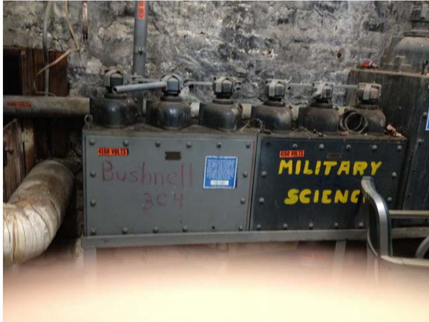
Military Science – Outdated 4160-volt switches.
