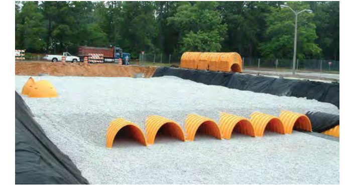
Example Underground Detention Basin
